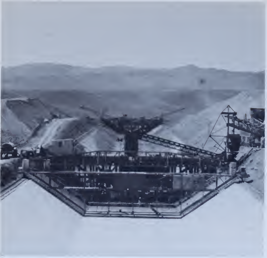
Figure 152. —A mammoth slip-form lining machine, with drop chutes, following the excavator—Delta-Mendota Canal, Central Valley project, California. DM-762-CV.
